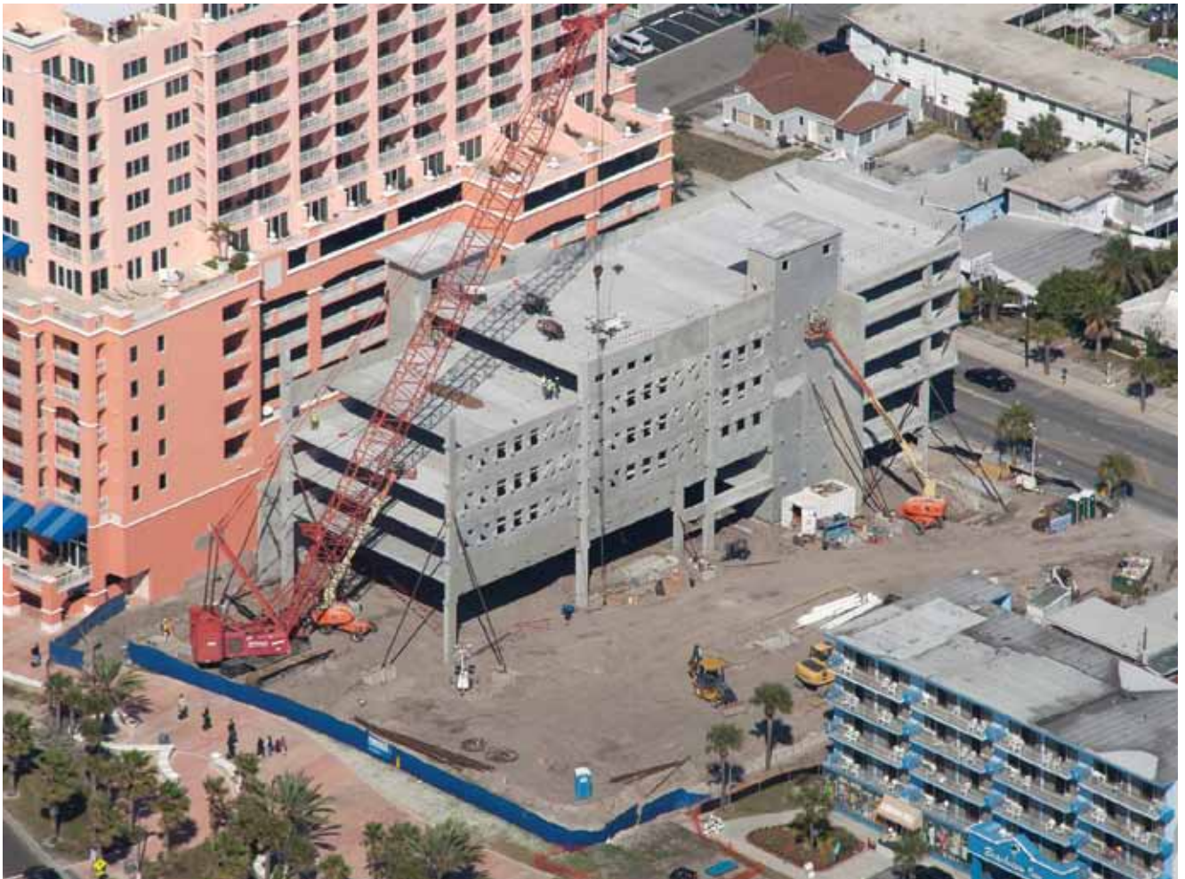
The tight site and busy area required the erection to be done almost entirely from within the building's footprint. Precast concrete components were shipped directly to the crane, where they were picked from the trucks to minimize disruptions. Photo courtesy of Aero Photo.
